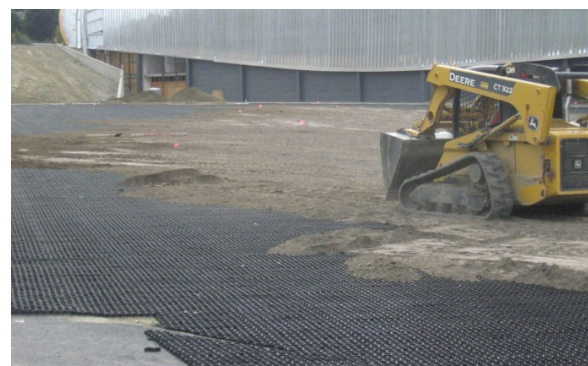
Using a heavy tracked loader to spread sandy loam filling the cells of EZ Roll grass paver.
