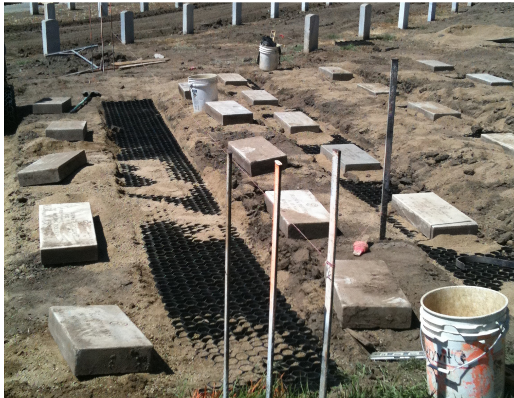
Above Photos: Installation of NDS EZ Roll Grass Paver for ground stabilization.
