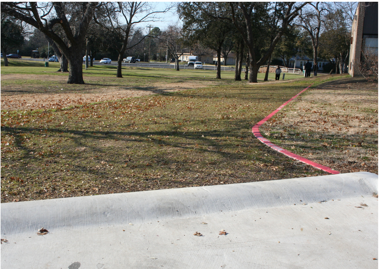
A picture of the site seven months after installation. The area is delineated with low-profile red curbing to mark the boundaries of the reinforced ground.
