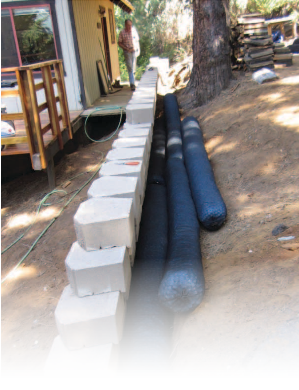
Jim Solomon at his cabin in Camp Nelson during the EZflow Installation.
