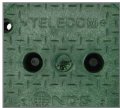
TELECOM marking on cover
